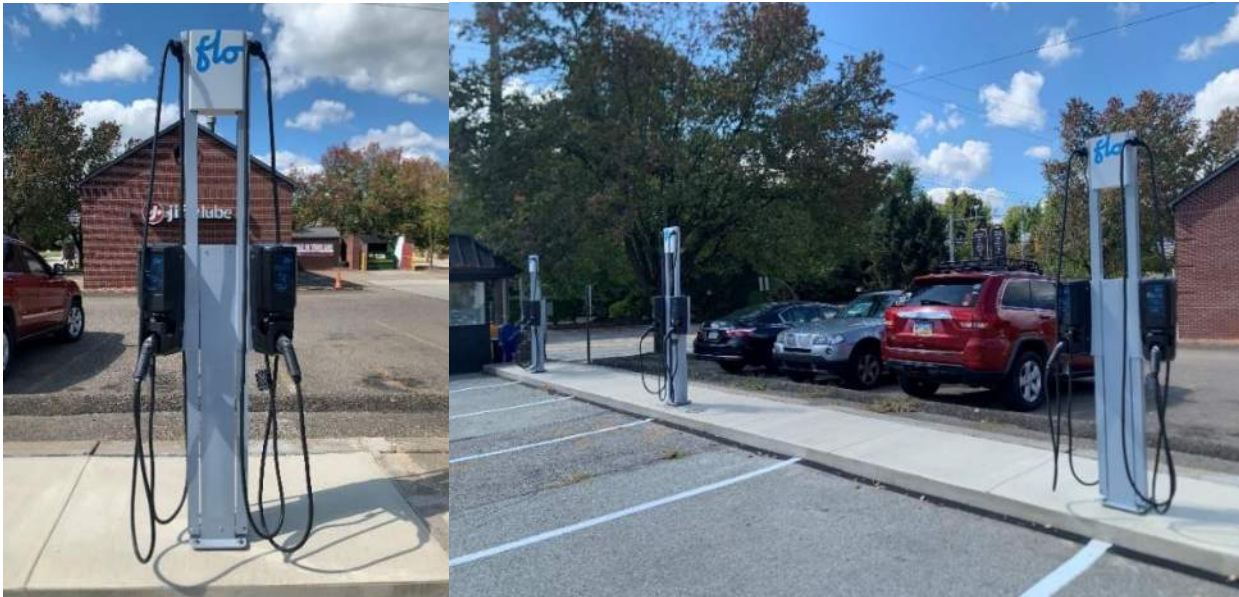
Figure 14: EV Charging Stations
